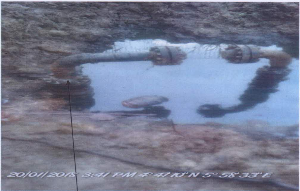
Spill Leak Point Before Repairs.
